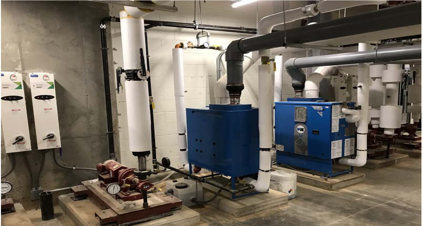
December 29, 2017 Mechanical Room
