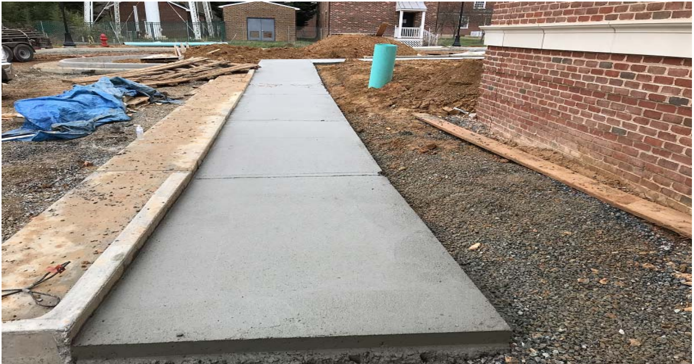
March 27, 2018 South Side Sub-Sidewalk at Handicap Parking
